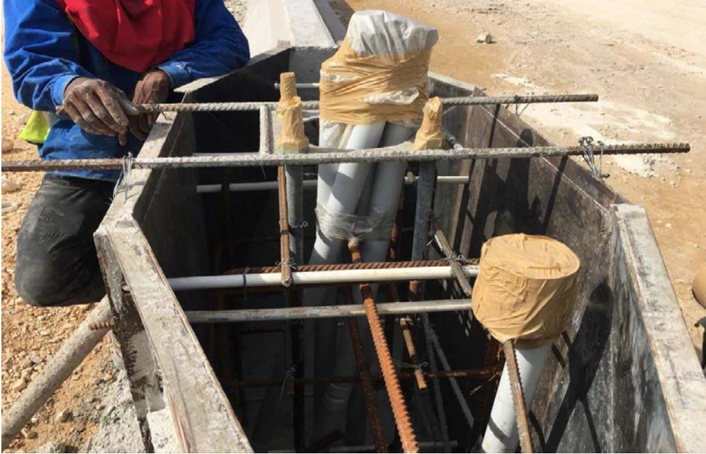
JPS Streetlight pole foundation
