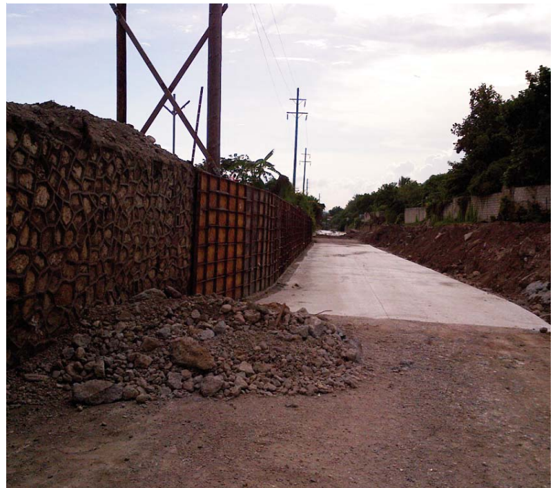
A section of the Gully Wall and Invert that are being re-established near the Washington Courts Apartments, St. Andrew
