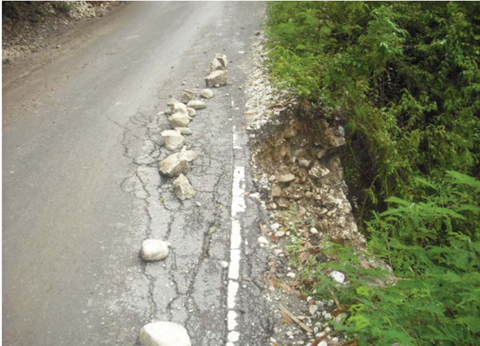
Roach Gully break away
