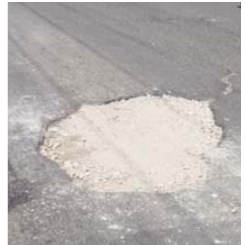
A typical pothole that has been prepared for Spray Patching
