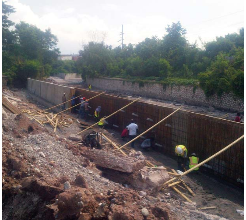
Workmen erecting Form work in preparation for the pouring of concrete for a section of the gully wall underway near Price Mart on Red Hills Road
