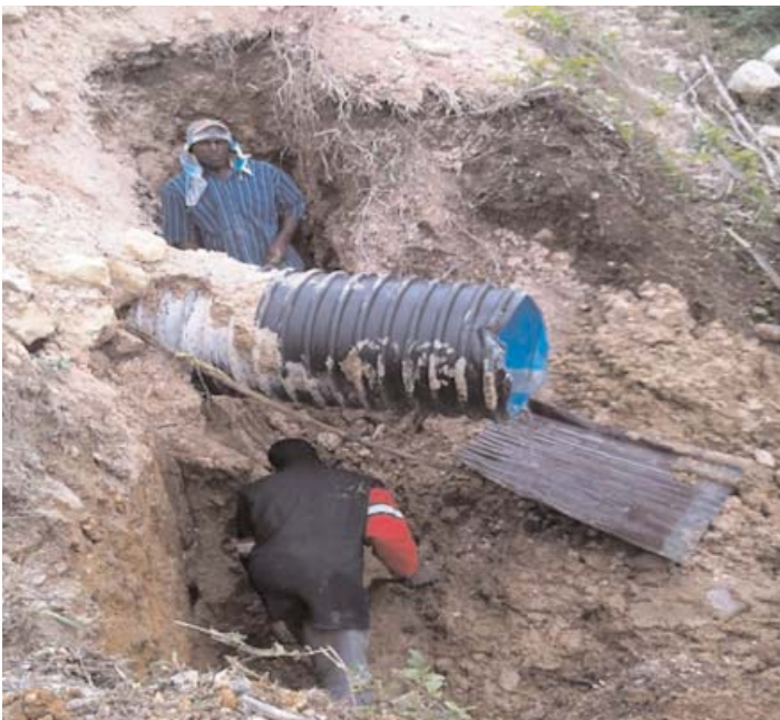
Wait-a-bit - Joe Hut Excavation work in progress for the construction of a Retaining Wall
