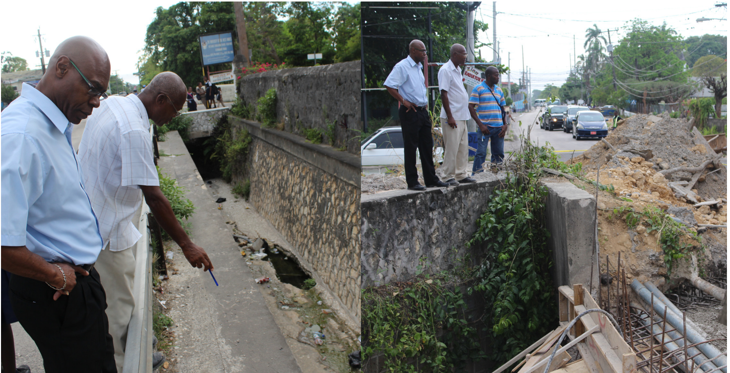
Mr. Hunter (1st left) on site at Fern Gully where the NWA is now in the final stages of completing an over $20 million dollar road and drainage improvement project.
