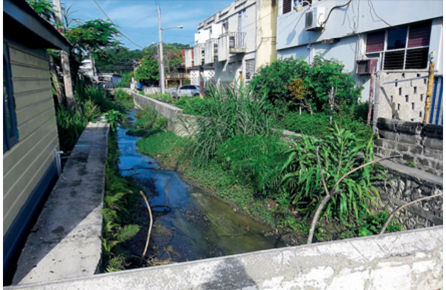
The Venture Gutter, which is the main drain which runs through the town of Lucea Hanover, is being targeted under the NWA's mitigation programme.
