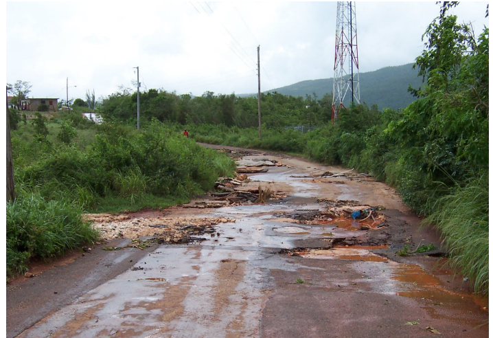
A section of a deteriorated road similar to those the NWA will be targeting for rehabilitation
