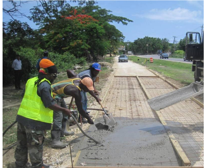
A view of the shared user path which is being constructed along the Norman Manley Boulevard in Negril, Westmoreland.
