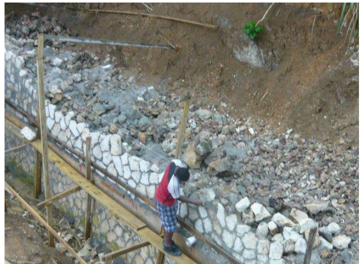
A section of the water way in Morgan's Bridge in Westmoreland where a retaining wall is now being constructed.
