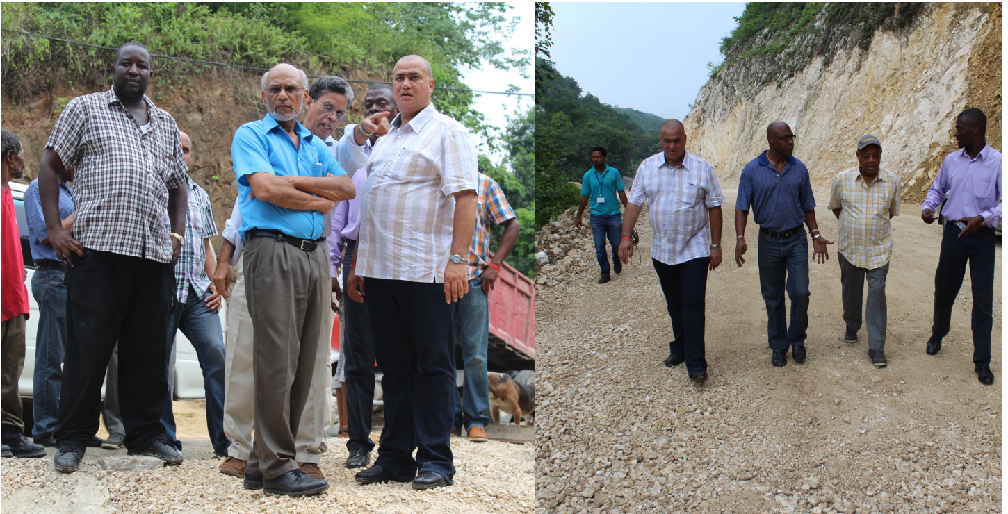
Minister Azan (right), on a site visit to John's Hall, St. James. The Agency is spending over $600m to re-align a section of the road and replace a bridge in the community. The project is to be completed by the end of the 3rd quarter of 2013\14.
