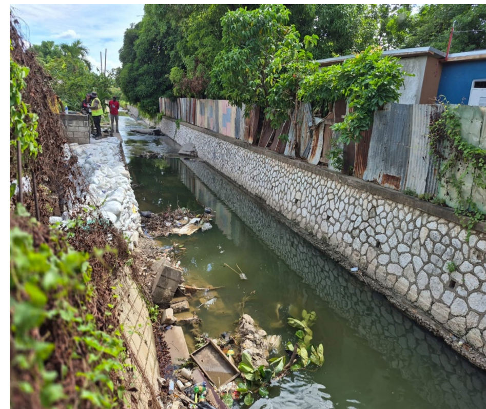
A gully in the corporate area where individuals have dumped garbage
