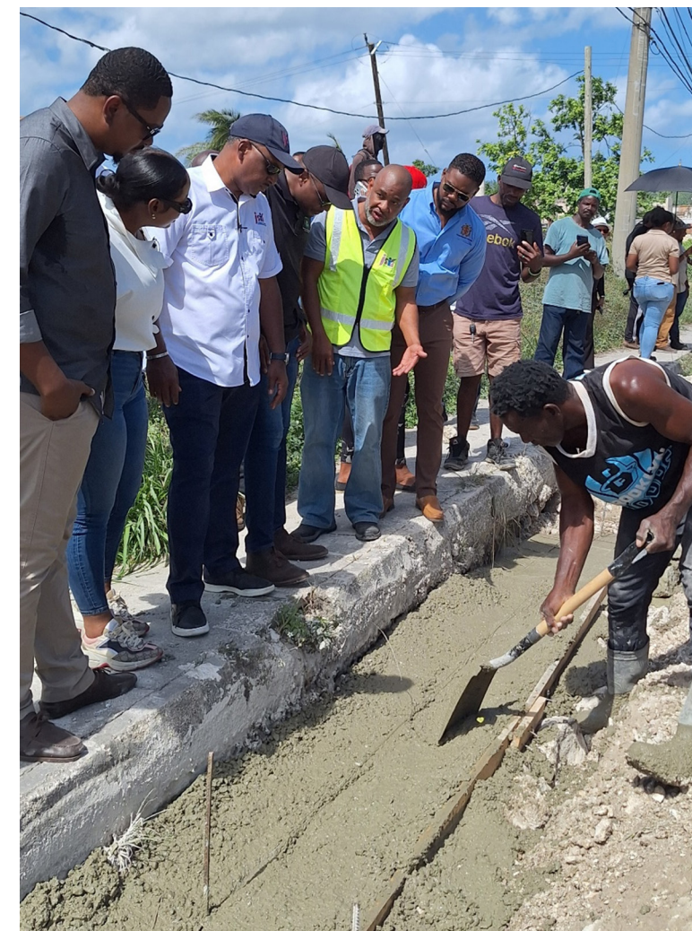
During a recent tour of the Montpellier roadway in St. James, Minister Robert Morgan as well as other members of the touring party observed works to construct a V-drain along a section of the corridor
