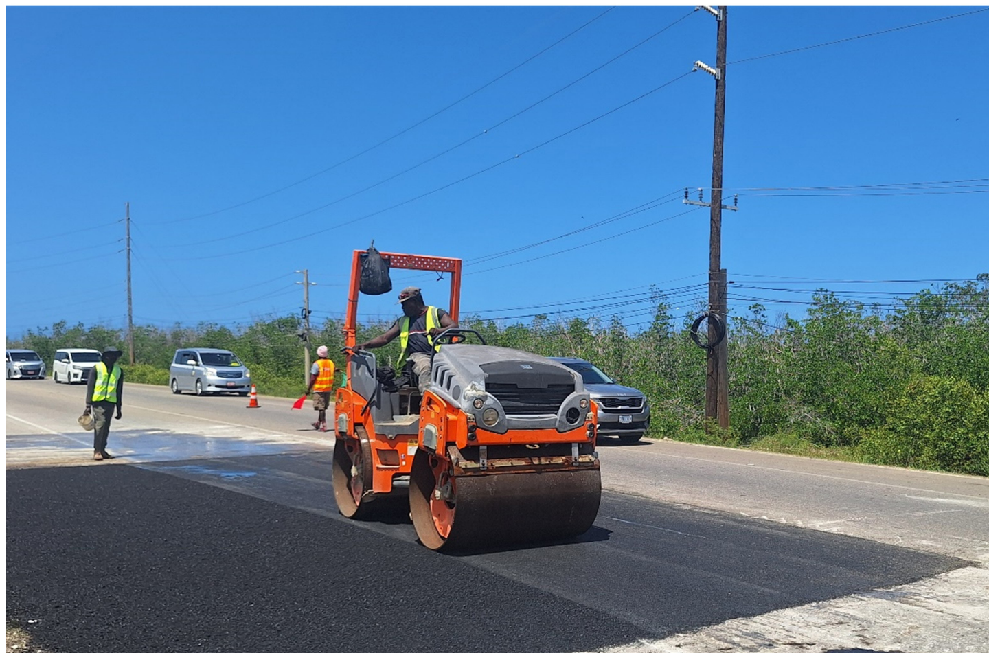
Patching works along a section of the North Coast Highway in Trelawny in the vicinity of the Greenside community.
