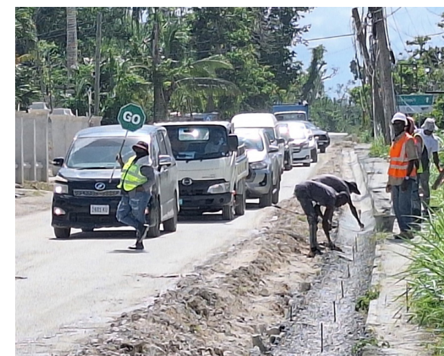
Construction of a V-drain along a section of the Montpellier roadway in St. James.
